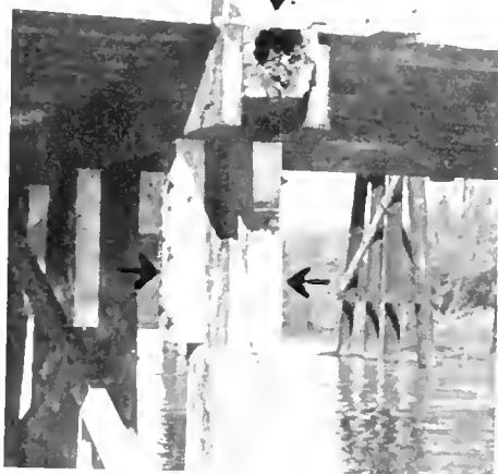
Pictures show typical repairs to a timber trestle scheduled for replacement in fall of 1943. Arrows point to rotted stringer and 6- by 8-inch corbels or supports bolted to the sides of the piles. The corbels support 4- by 16-inch stringers used to reinforce the cap
